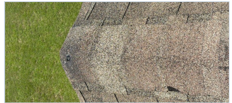
9. Second damaged ridge cap at the hip corner with an exposed fastener.
