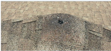
10. Plumbing penetration requiring a rain collar, with granule loss around the penetration.
