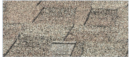
6. Close view of the shingle surface showing granule loss and wear across the field.
