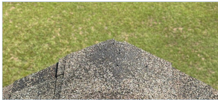
8. Damaged ridge cap shingle with exposed fasteners at the cap.
